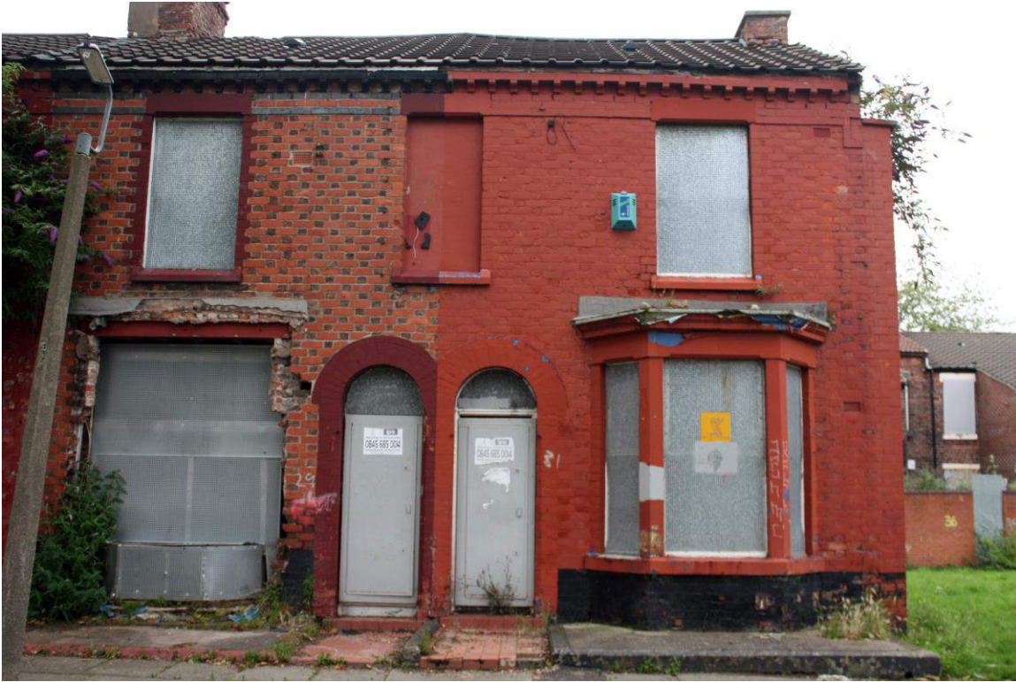
The house on the right was in good condition when it was requisitioned for clearance, and has since deteriorated due to lack of drainpipes and maintenance.
